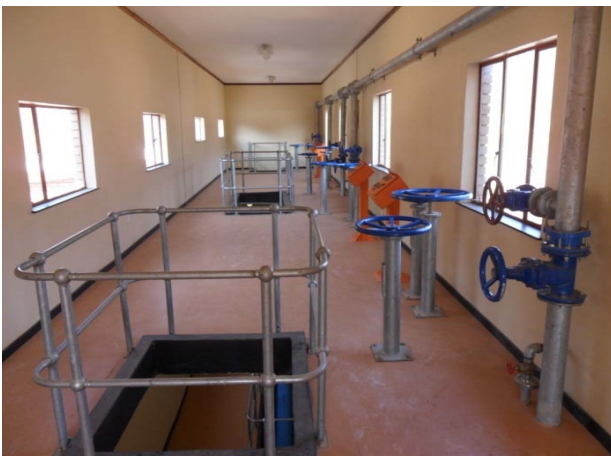
Pictures of Mutshedzi Water treatment plant
