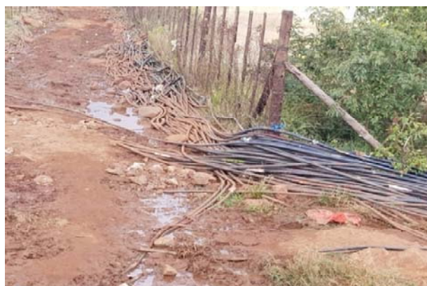
Illegal connections in raliphaswa village Nzhelele
